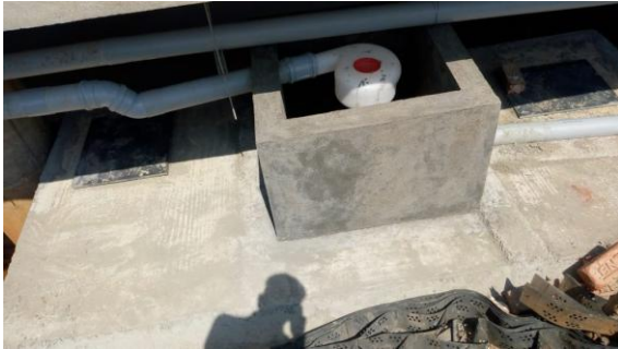
Pipes run along the cellar ceiling.
